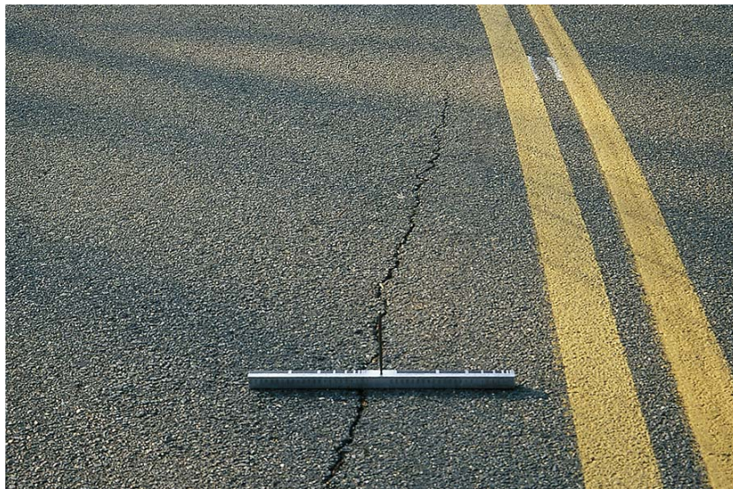
Figure 13 - High Severity Longitudinal Cracking not in Wheel Path
