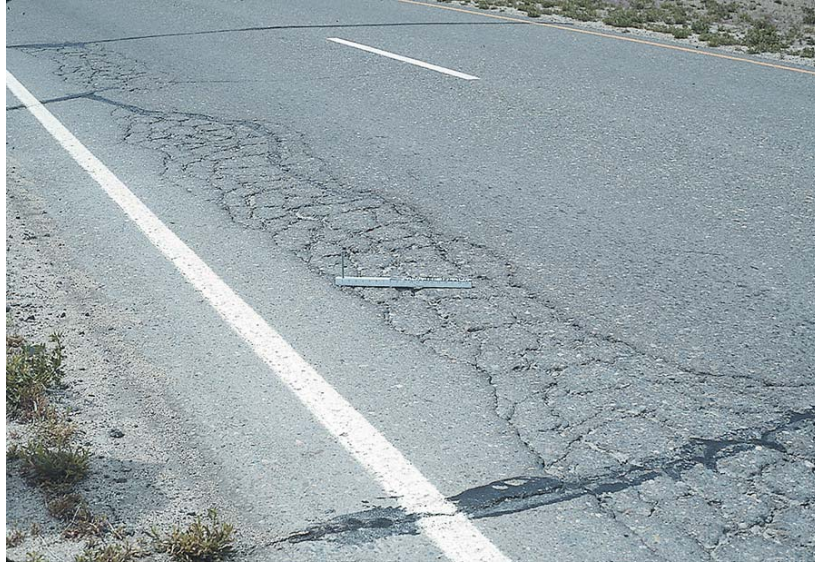
Figure 5 - High Severity Fatigue Cracking with Spalled Interconnected Cracks
