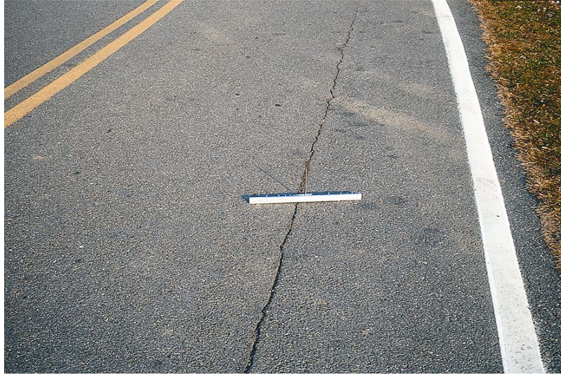
Figure 12 - Moderate Severity Longitudinal Cracking in the Wheel Path
