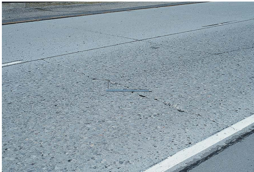
Figure 44 - High Severity Transverse Cracking
