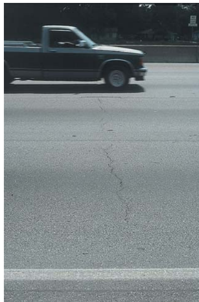
Figure 17 - Low Severity Transverse Cracking
