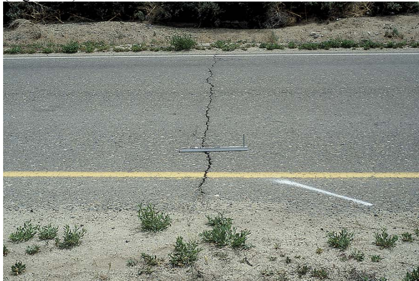
Figure 19 - High Severity Transverse Cracking
