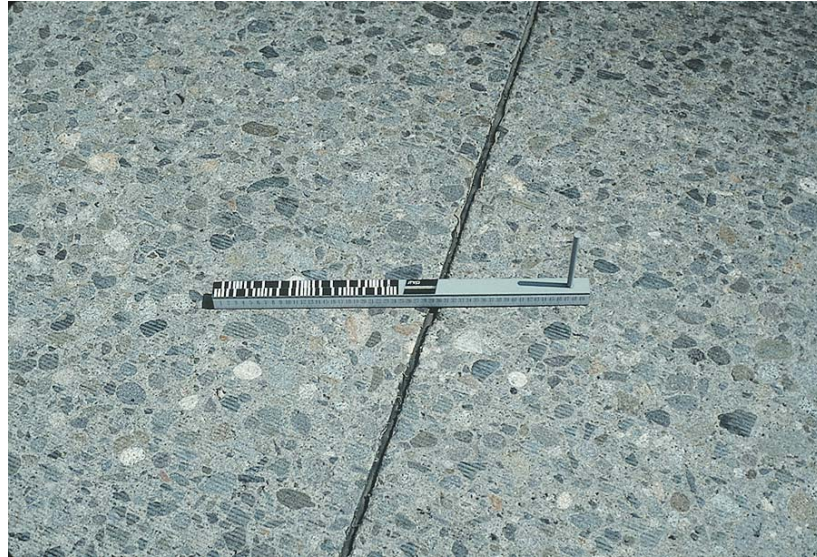
Figure 45 - Low Severity Joint Seal Damage
