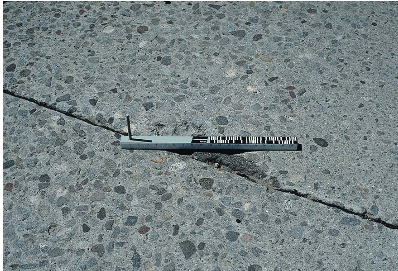
Figure 51 - Moderate Severity Spalling of Transverse Joint, Close-up View
