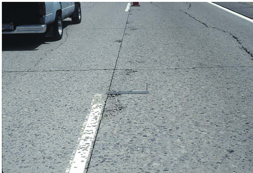
Figure 48 - High Severity Spalling of Longitudinal Joint
