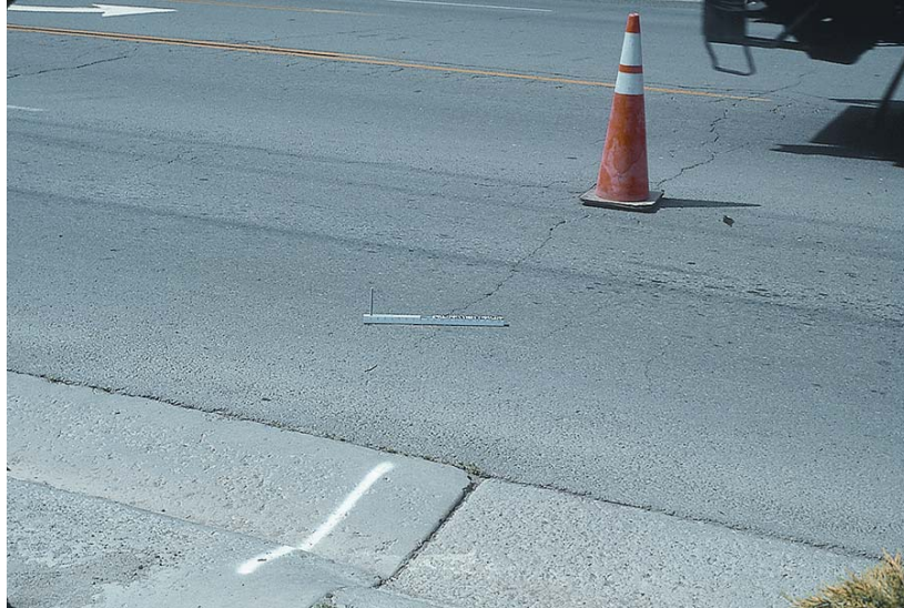
Figure 18 - Moderate Severity Transverse Cracking
