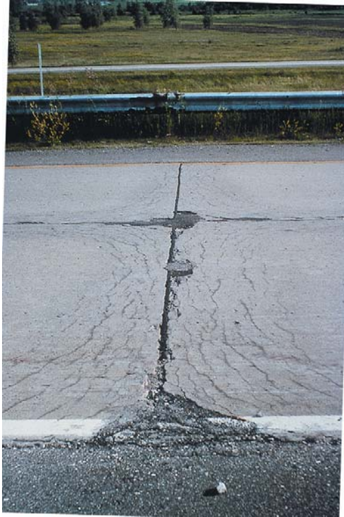
Figure 37 - High Severity “D” Cracking with Loose and Missing Material
