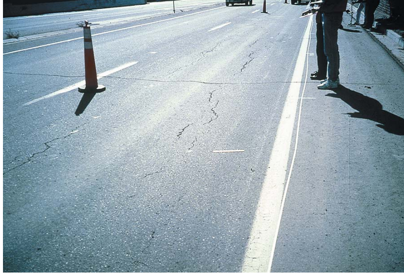
Figure 3 - Low Severity Fatigue Cracking
