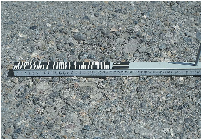
Figure 31 - Loss of Course Aggregate
