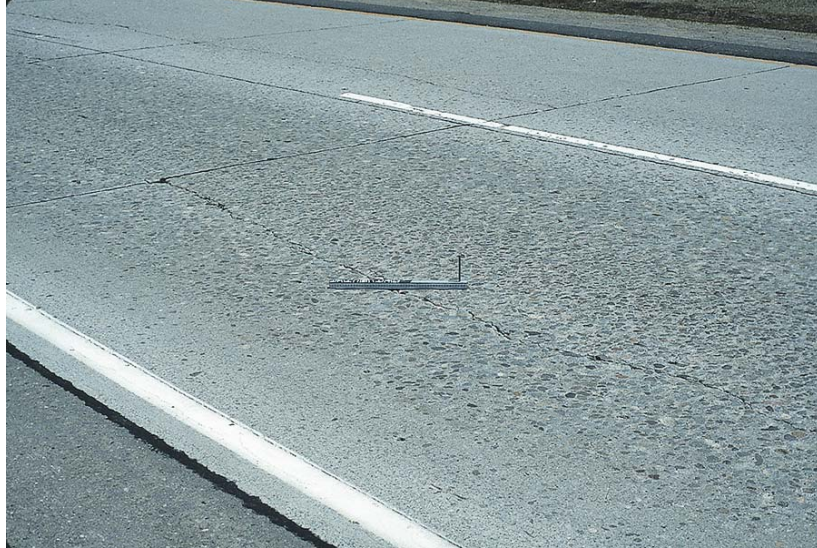
Figure 40 - Moderate Severity Longitudinal Cracking
