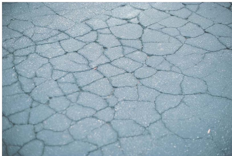
Figure 2 – Chicken Wire/Alligator Pattern Cracking
