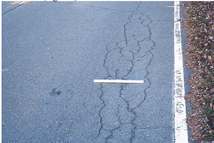
Figure 4 - Moderate Severity Fatigue Cracking
